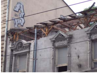
Ancient wood (log) columns and rafters get exposed during a restoration project. Strict compliance with restoration and historic site preservation codes make for a strange blend of modern conveniences and old structure systems.
